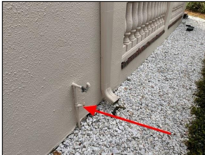
Main water shutoff valve
