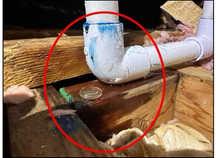
Water damaged framing & ceiling
