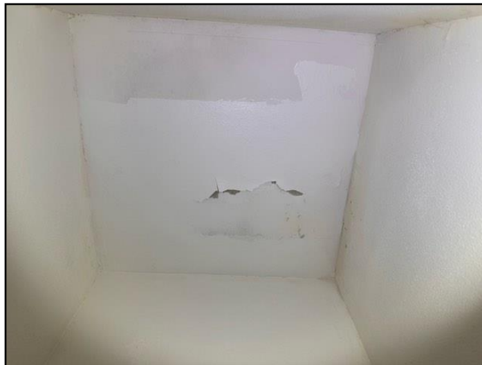
Paint peeling inside closet 2nd floor hallway
