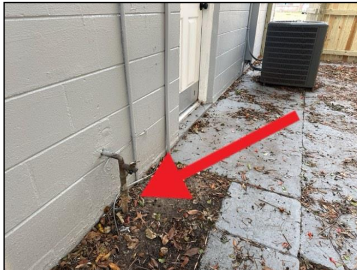
Main water shutoff valve
