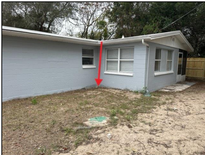
Gutter splash shield missing
