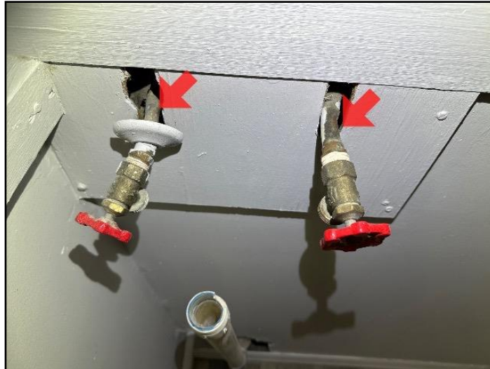
Pipe damaged- requires repair
