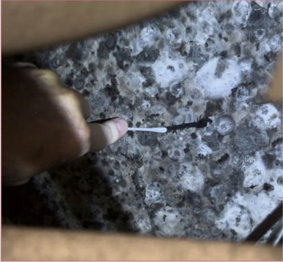
Actual sample location in air handler All insulation must be replaced, mold CANNOT be cleaned from this material
