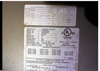
Air Handler Manuf: 2015
