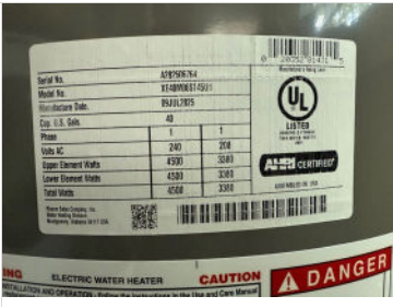
Water Heater Manuf: 2025
