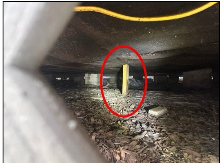
Multiple single board supports present
