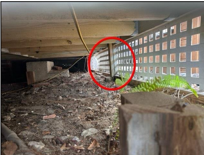
Multiple perimeter supports are wood in soil
