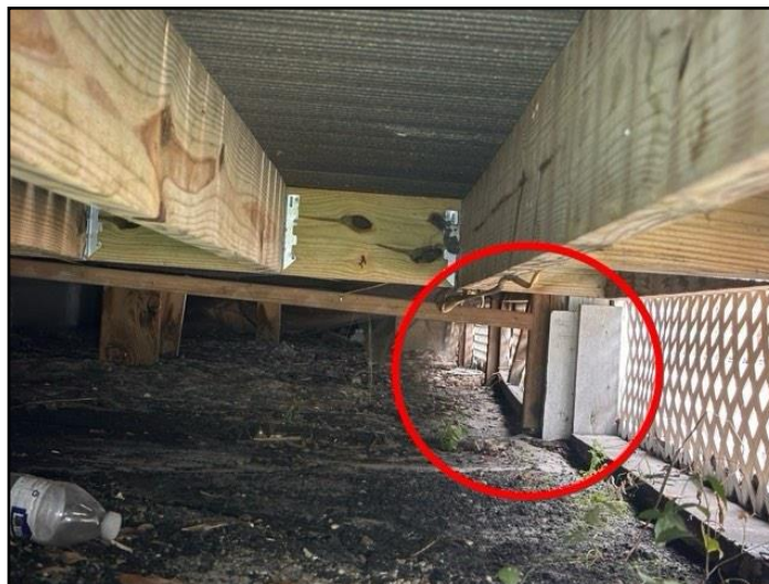
Multiple perimeter supports are wood in soil
