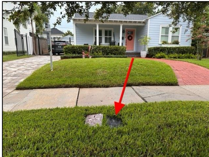
Main water shutoff valve
