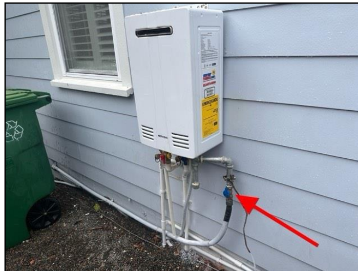
Water heater gas shutoff valve
