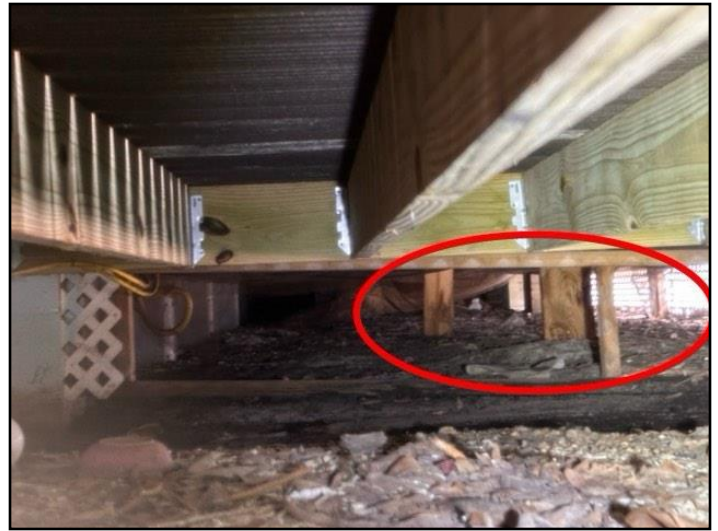
Multiple single board supports present
